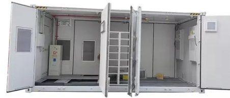
1075KW HH ESS
